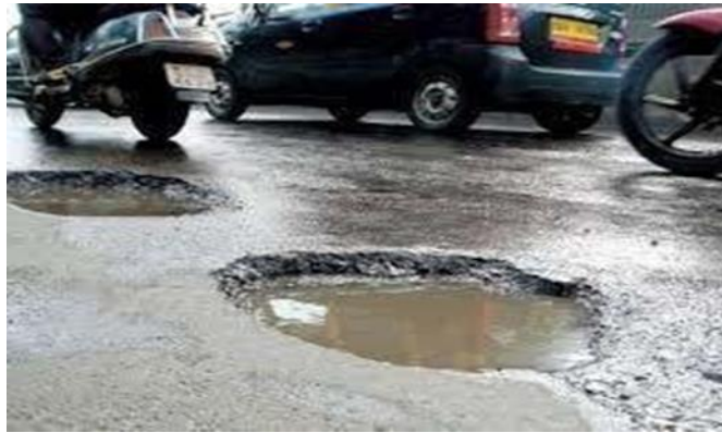
Fig. 1. Condition of roads with potholes.
