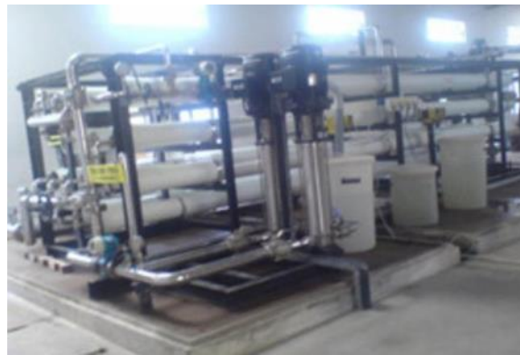
Fig:3 Reverse Osmosis plant
