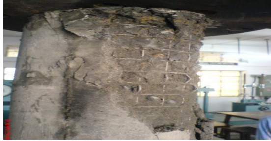
Figure: 4 Failure of weld mesh confinement
