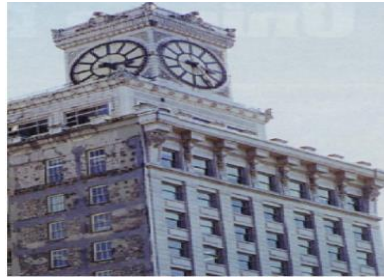
Figure 1: The north and west elevations of the Vancouver Block Building before the rehabilitation works.
